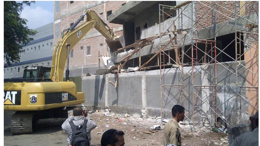
Figure 2. Jakarta City Government forcibly demolished the five-story building in East Jakarta due to land use violation and permit
